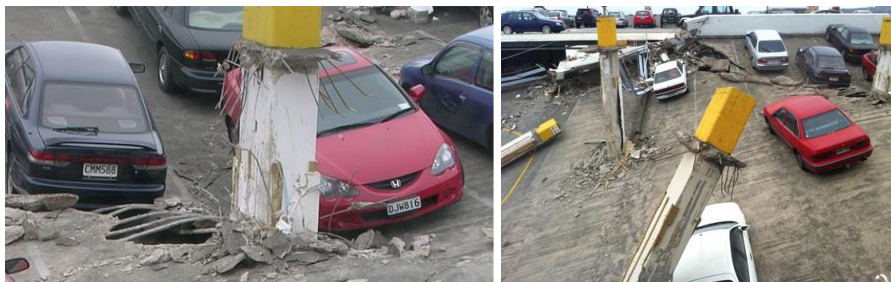
Figure C2G.2: Collapse of flat-slab system observed in Christchurch (from Kam et al., 2011)
