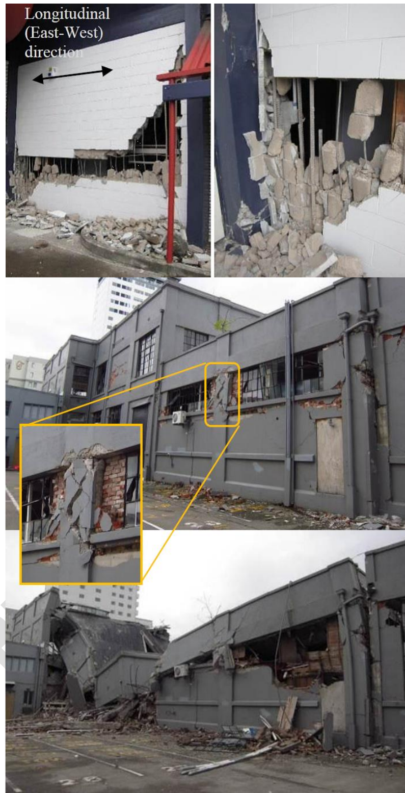
Figure C7.8: Masonry infill frame damage observed following the 2010–2011 Canterbury earthquakes (Kam et al., 2011)
